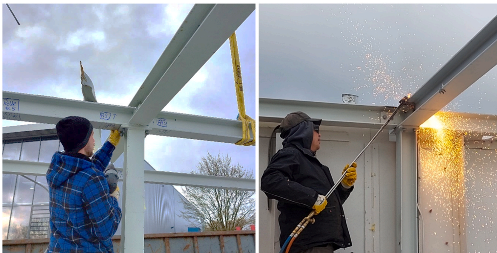
Fig. 5. Careful deconstruction of steel beams: Loosening bolted connections (left) and thermally cutting through beams (right).
